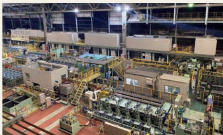
Steel bar processing (PM) line at Chita Second Plant
