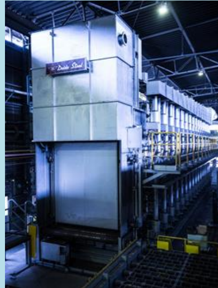
Premium STC® furnace, operating at our Hoshizaki Plant
