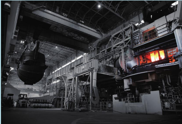
Electric arc furnaces with rotating drives(STARQ®) operating at Daido Steel's Chita Plant
