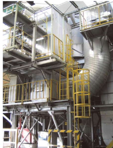
Fig. 14. View of heat recovery boiler.
