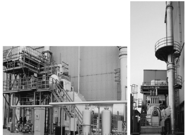
Fig. 11. View of heat recovery boiler
