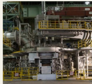
炉体旋回式電気炉 (STARQ®)
